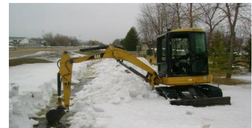
Taking snow out of ditches allows water to flow away in spring Photo from www.plowsite.com
