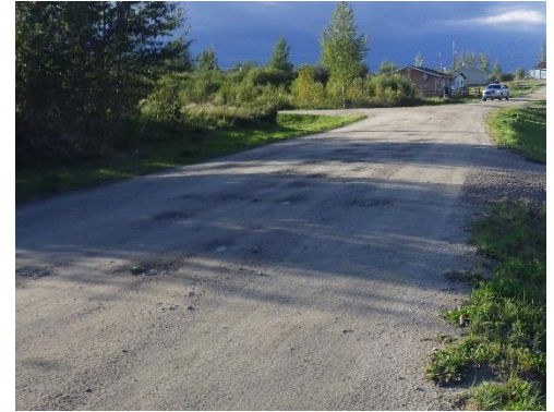
Dirt and gravel roads can become marked with potholes when water doesn't drain away properly.
