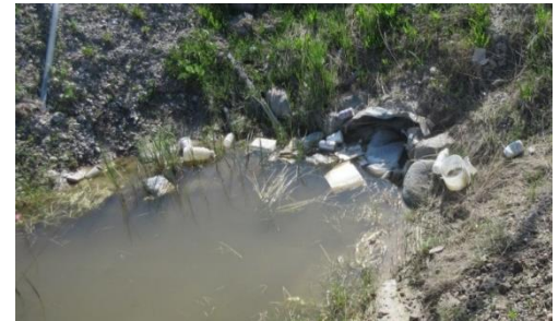
Damaged or blocked culverts and ditches can't carry water away like they should.
